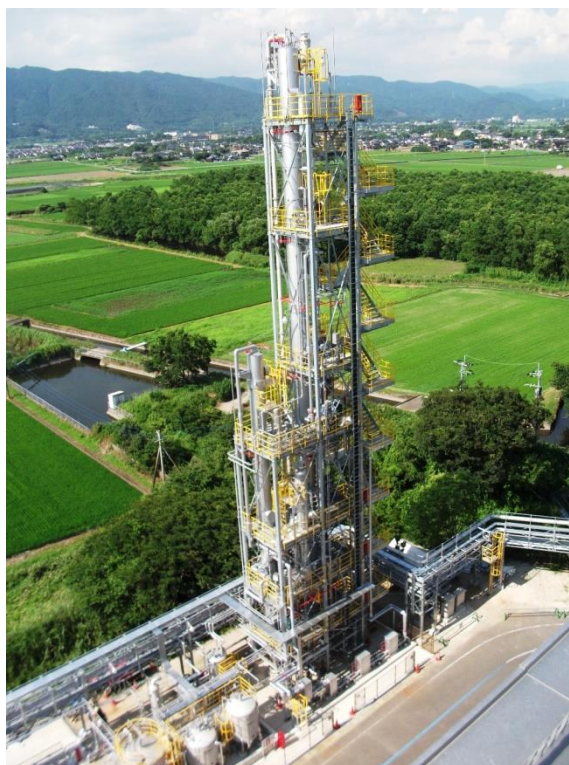
Fig. 4 10 tpd Capture Plant (Source: Toshiba web site 4 )
