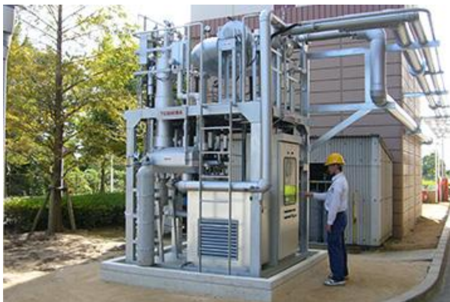
Fig. 3 10kgpd Capture Plant (Source: Toshiba web site 3 )
