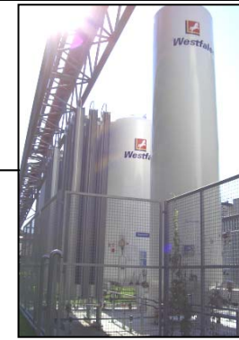
O 2 /CO 2 supply tanks
