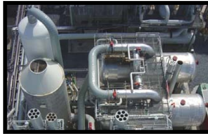
Air Cooling and Pretreatment
