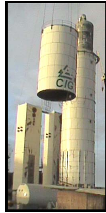
Field erected column can
