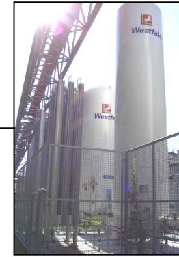
O 2 /CO 2 supply tanks
