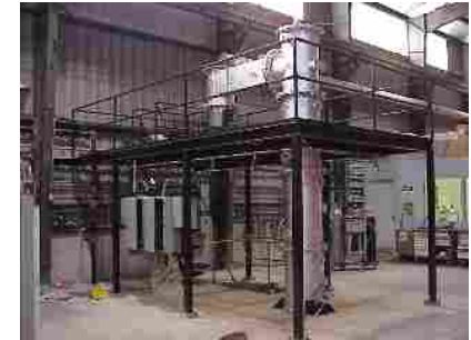
300 kW Circulating Fluid Bed
