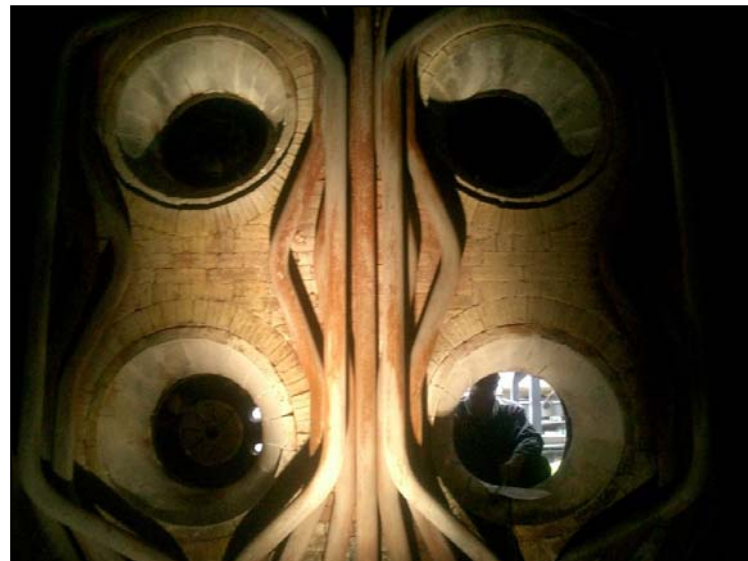
Openings for the four existing air-fired natural gas burners
