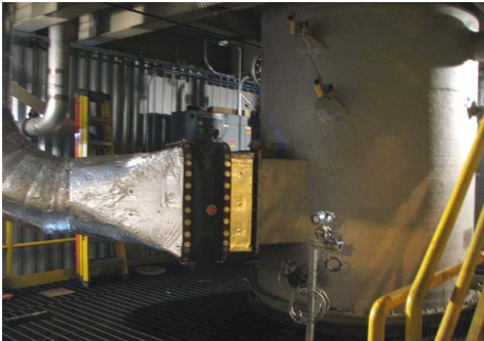
Tower Inlet Flue
