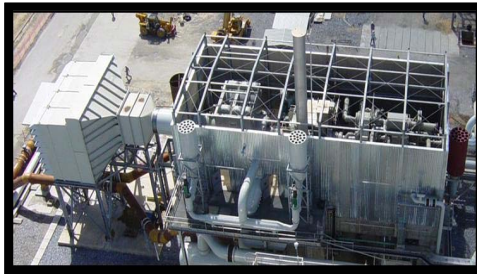
Main and Boost Air Compression
