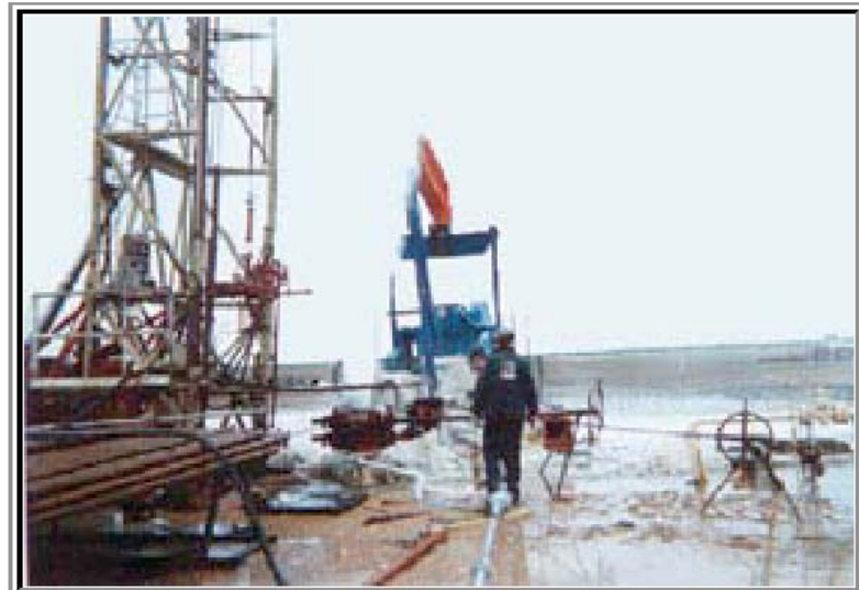
Fig. 4. Accumulation of dry ice and hydrates on the pump unit skid and gear box, plus 1 to 2 in. accumulation on the ground.
