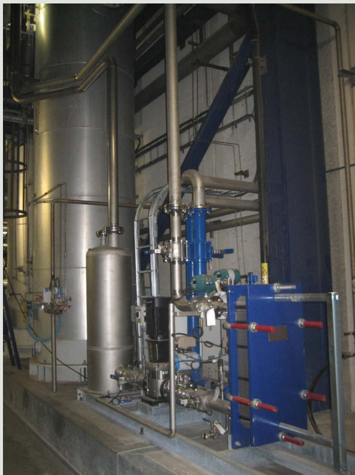
Absorber inter-cooler skid
