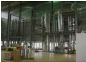
E.ON Karlshamn Sweden - 5 MWth Chilled Ammonia - Fuel/Gas
