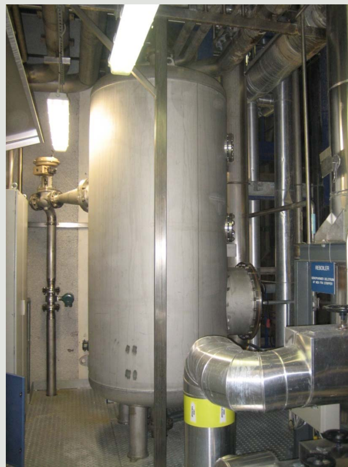
Flash vessel for vapour recompression
