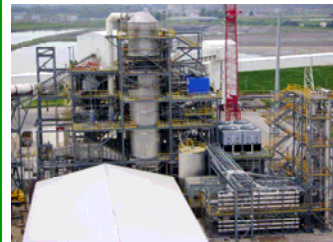
AEP Mountaineer USA - 30 MWth Chilled Ammonia - Coal
