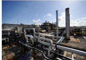
Total Lacq France - 30 MWth Oxy - Gas/Fuel
