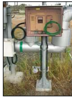
CO 2 detector (No leak)
