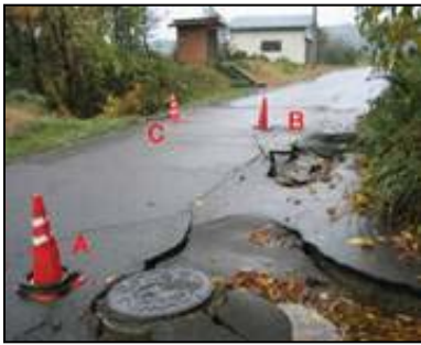
Access road was damaged.
