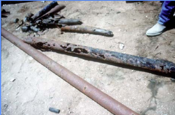
Leaking pipe retrieved
