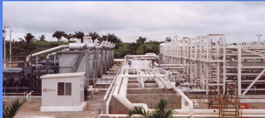
CO 2 EOR Facility in Carmito, Mexico Separates, Compresses, Distributes CO 2
