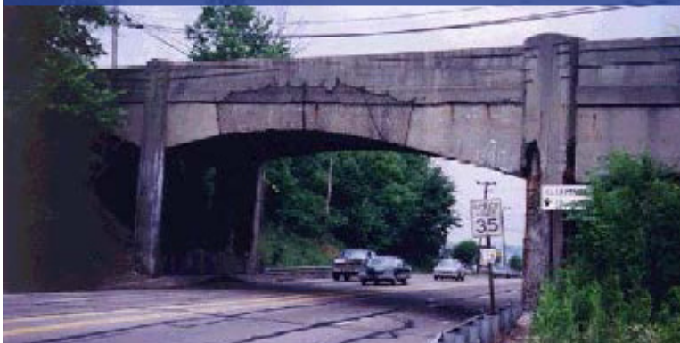
Two examples of cement structures, one that has suffered corrosion, and one that has withstood the elements; illustrative of the extremes of cement composition and endurance
