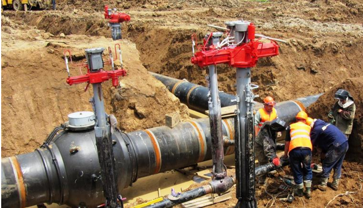
Figure 13 – Example of typical block valve in natural gas pipeline (Gazprom, 2011)
