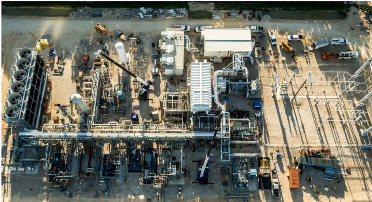
La Porte Demonstration Facility – April 2017
