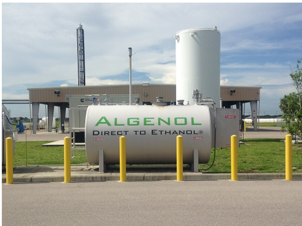
Figure 4.9 Ethanol storage tank with ethanol separation facility in background
