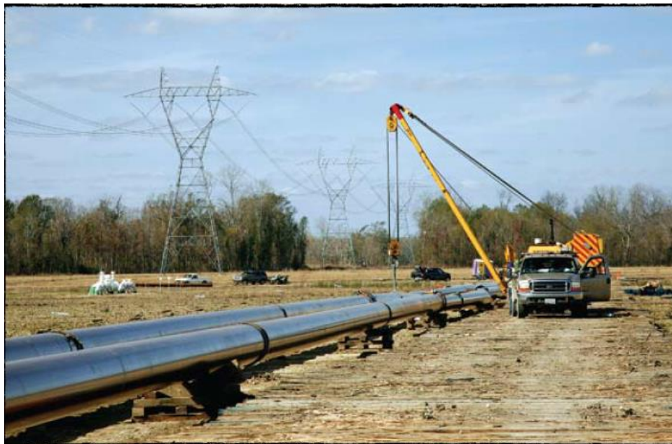
Figure 28: New dedicated CO 2 pipeline the Green Line built by Denbury to collect anthropogenic CO 2 from sources in Louisiana and Texas and integrate them with the natural source of CO 2 from Jackson Dome (Denbury Resources Inc., 2008).
