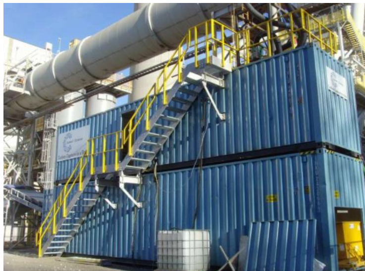
Figure 9-2: Photograph of the CO 2 ntainer unit developed by Carbon8 installed at the Montalieu cement plant (Lyon, France) operated by Vicat (AggNet, 2021)
