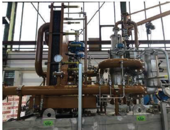
Oil lube unit
