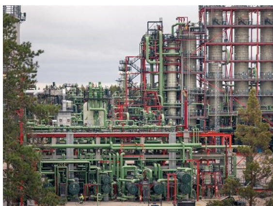
Porvoo Refinery, Finland
